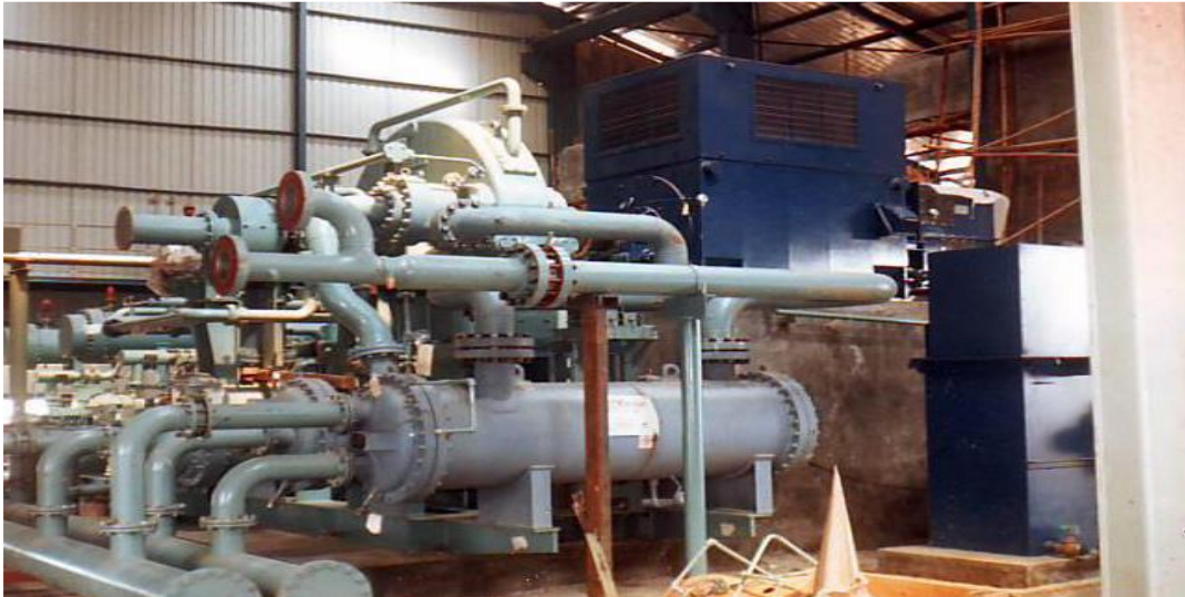
Gambar 5.1 Kompresor Udara ( Air Sparation Plant )
